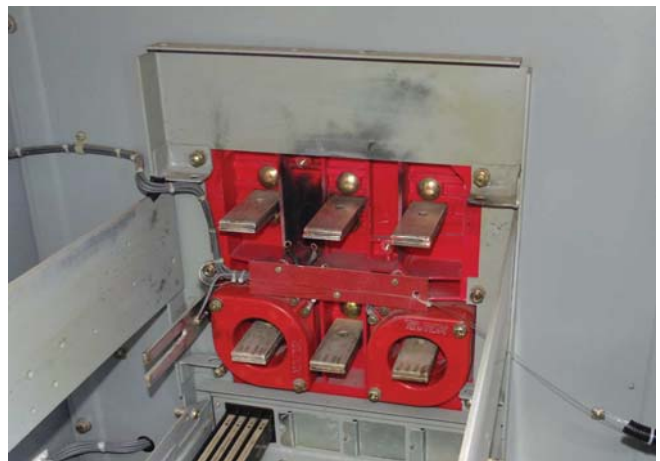
Fig. 10 Photo of damage to feeder compartment after arc fault with HSGS protection.
