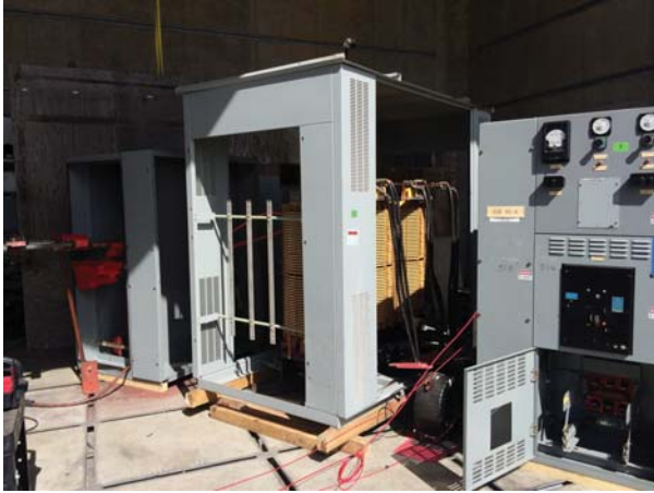
Fig. 4 Substation test arrangement.
